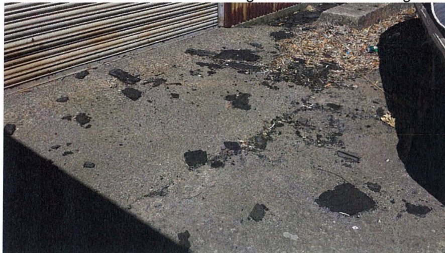
Roof Membrane Debris along West Wall of Building
