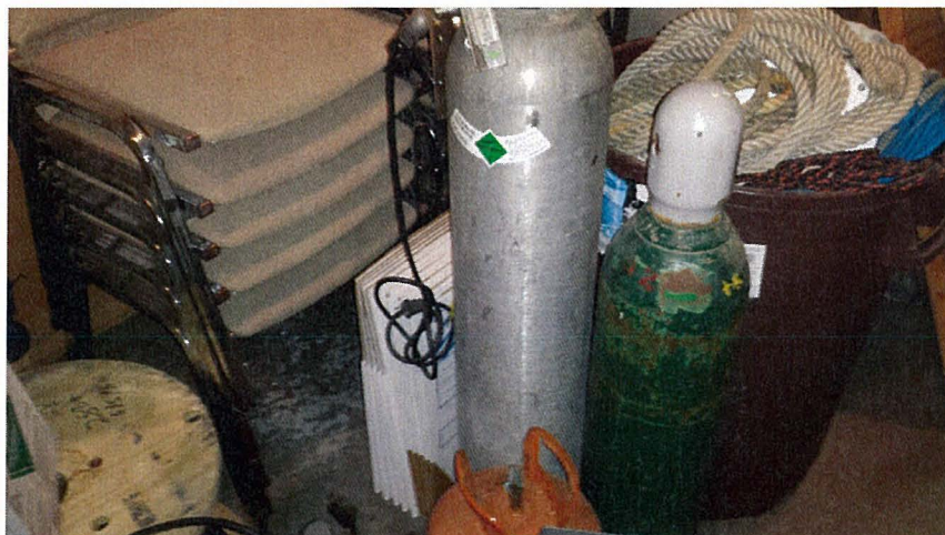
Unsecured Carbon Dioxide, Oxygen and unknown Orange Gas Cylinders
